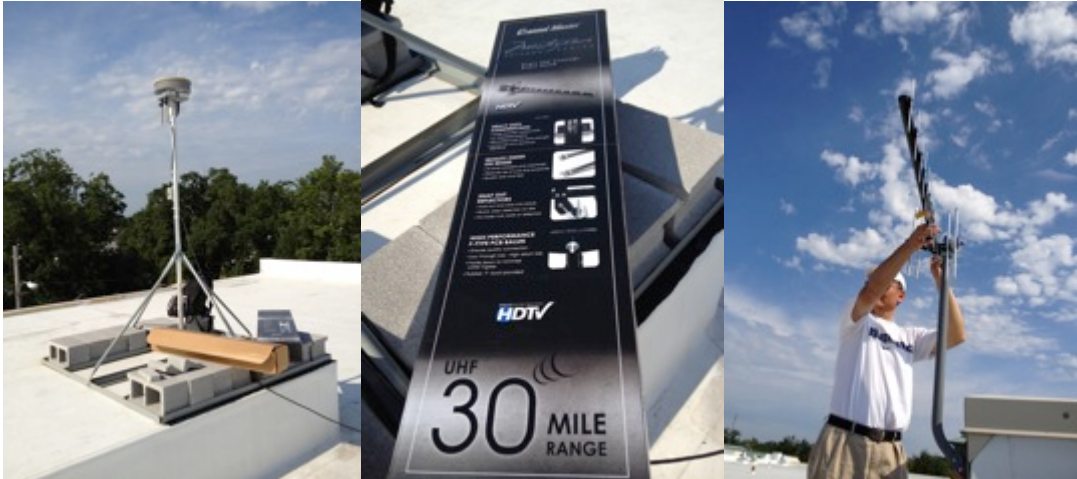
Figure 25: Cape Fear Museum Roof Antenna (source: William Edwards, 2012)
