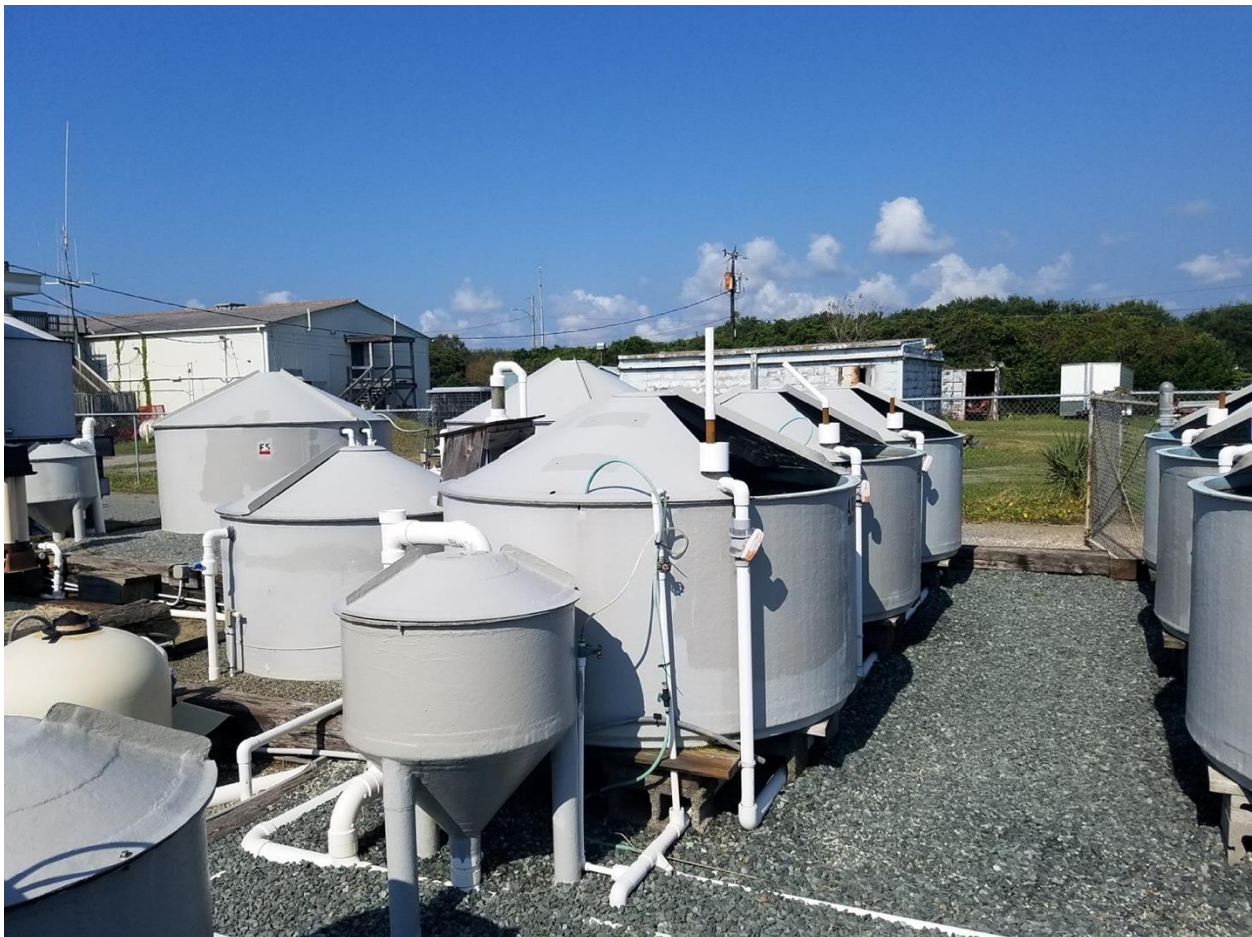
Figure 1 UNCW Aquaculture Research Facility
